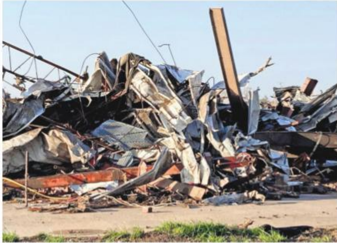
A structure torn up by the tornado in Rolling Fork, Mississippi on Saturday | AP
