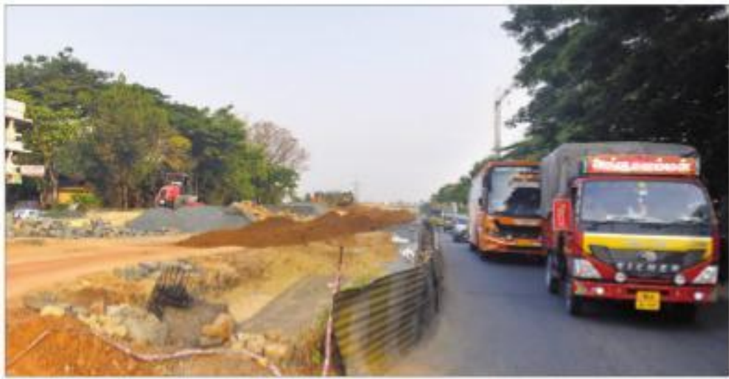
The construction work of Chalakudy bridge on NH-44 has reached the final phase | A SANESH
