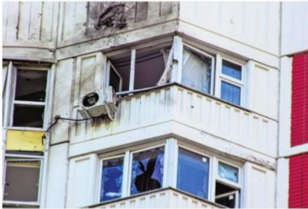
The image shows a damaged part of an apartment building which was attacked by an Ukrainian drone in Moscow, Russia on Tuesday | AP
